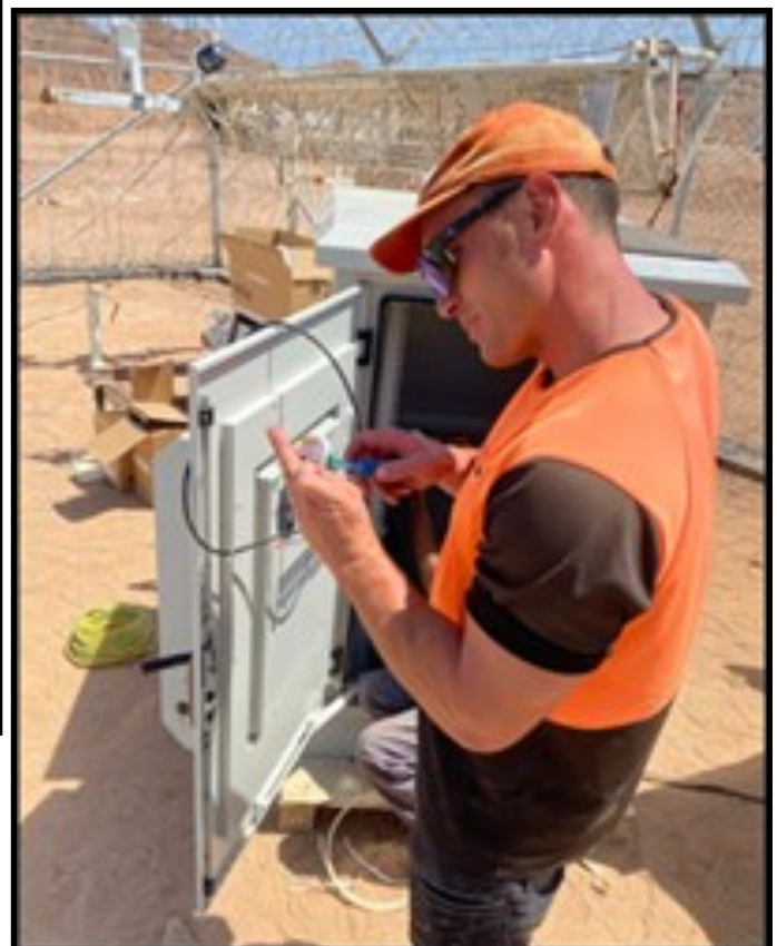
LCPL Te Heu Heu (NZ Army Electrician) consistently out in the hot Sinai sun getting the power back up.
